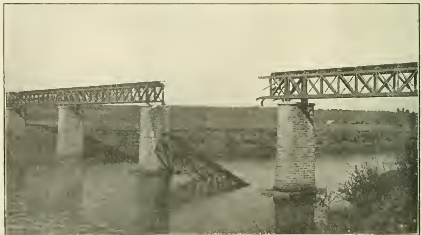
VAALE RIVER BRIDGE. CENTER SPAN THROWN DOWN DURING THE BOER WAR.
